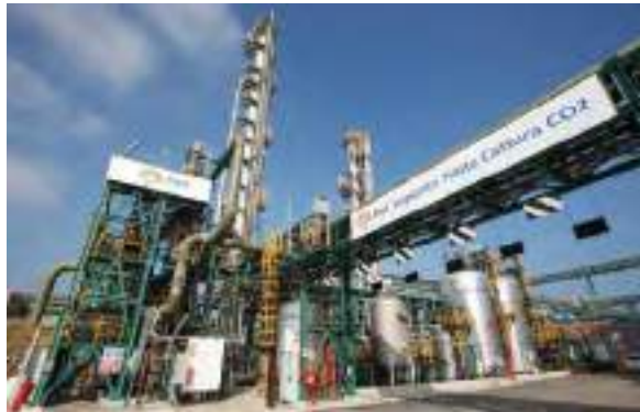
CO 2 capture plant at the 2 600 MW Brindisi Sud coal-fired power plant operated by ENEL in Italy
